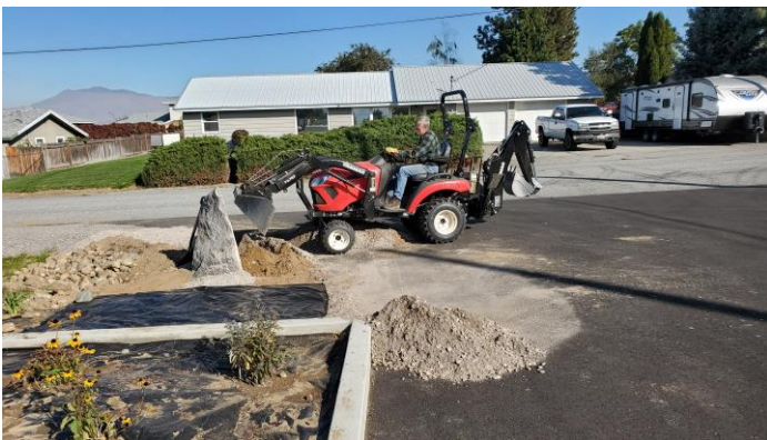
Rowe's tractor and backhoe made life MUCH easier for everyone. Thank you neighbor, Rowe's Tractor, for the 50% discount for a week's rental!!! Driver, Chuck St. John.
